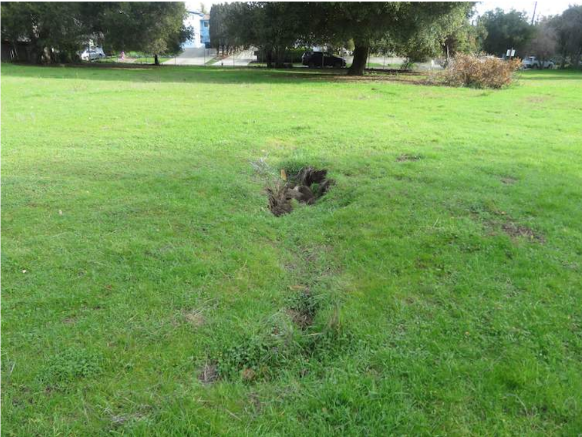
Photograph 8 – Area of subsidence.
