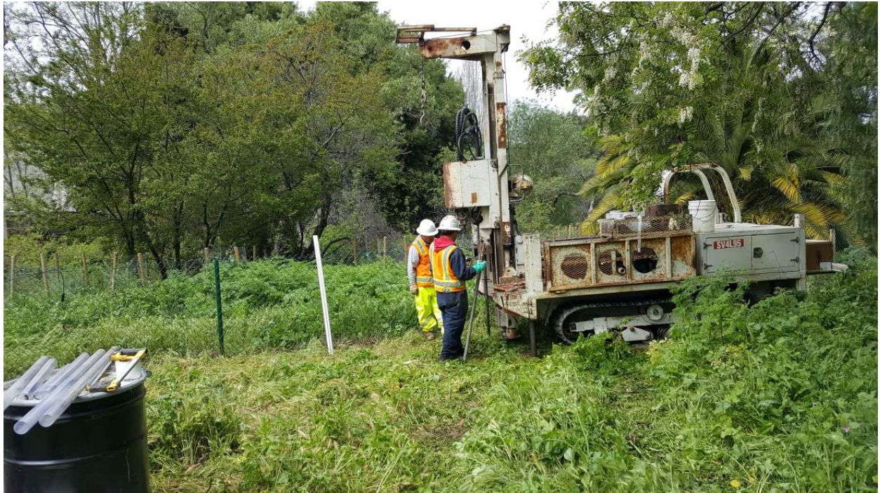
Photo 4: View of bore SB-1 being prepared for advancement using narrow access drill rig, looking west.
