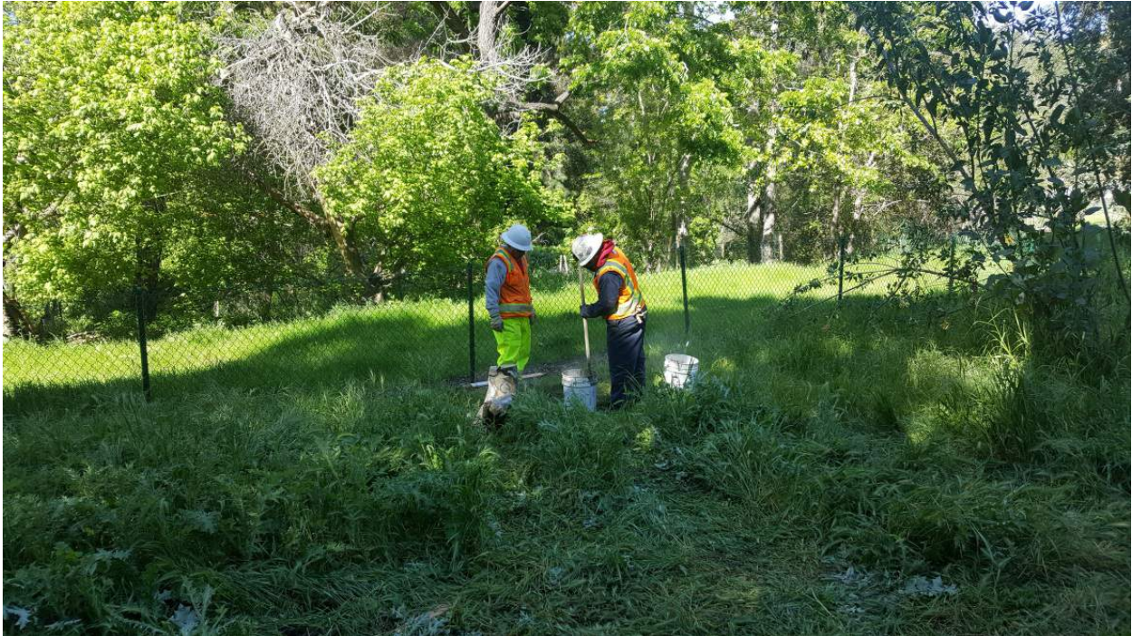
Photo 9: View of bentonite slurry being prepared prior to closing SB-6, looking west.
