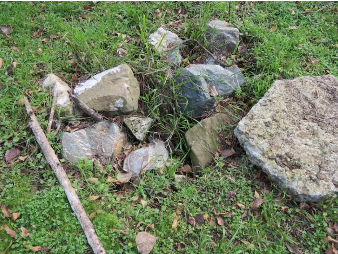
Photograph 12 – Area of subsidence.
