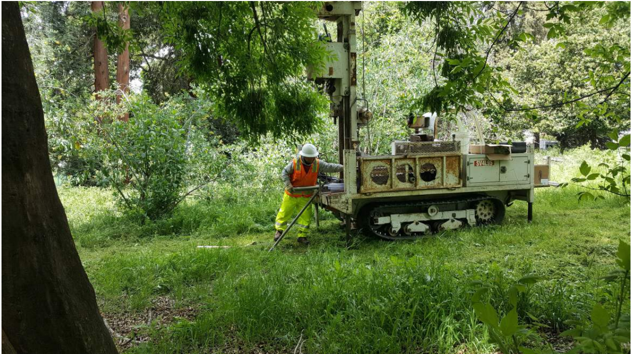
Photo 6: View of narrow limited drill rig being maneuvered into position prior to advancing SB-4, looking north.
